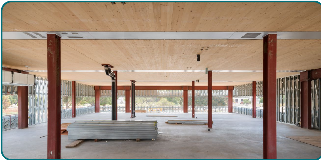
Construction progress photo. Open laboratory environment with mass timber technologies. Photo: HDR, Inc.
